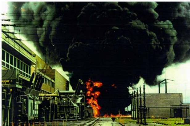
Fig. 1: Transformer fault due to a defective bushing
