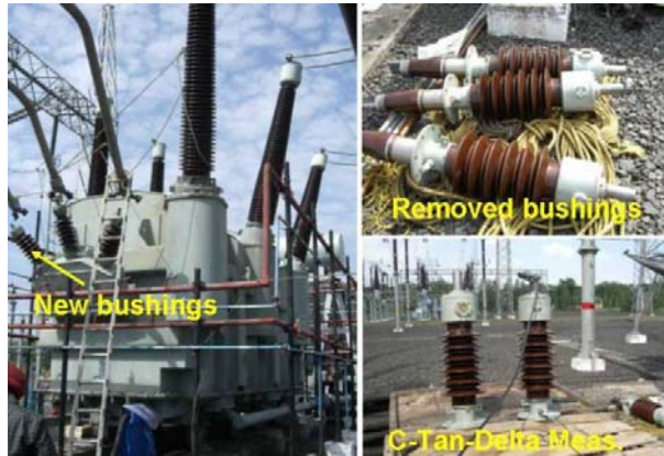
Fig. 21: 33kV OIP bushings
