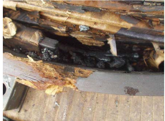
Fig. 15: Defective winding with interrupted conductors
