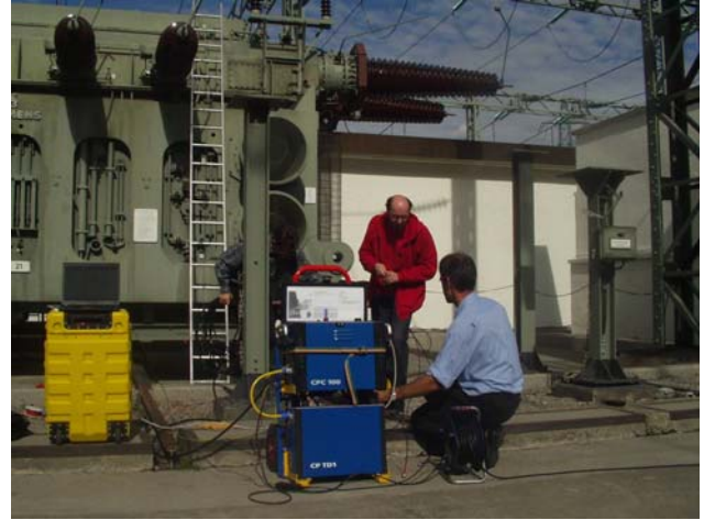
Fig. 10: Impedance measurements on defective transformer
